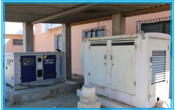
STAND BY GENERATORS
