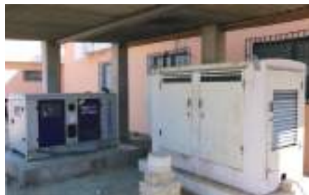
STAND BY GENERATORS
