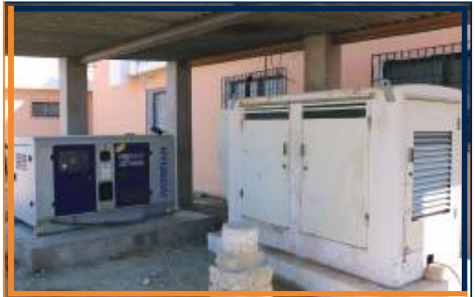
STAND BY GENERATORS
